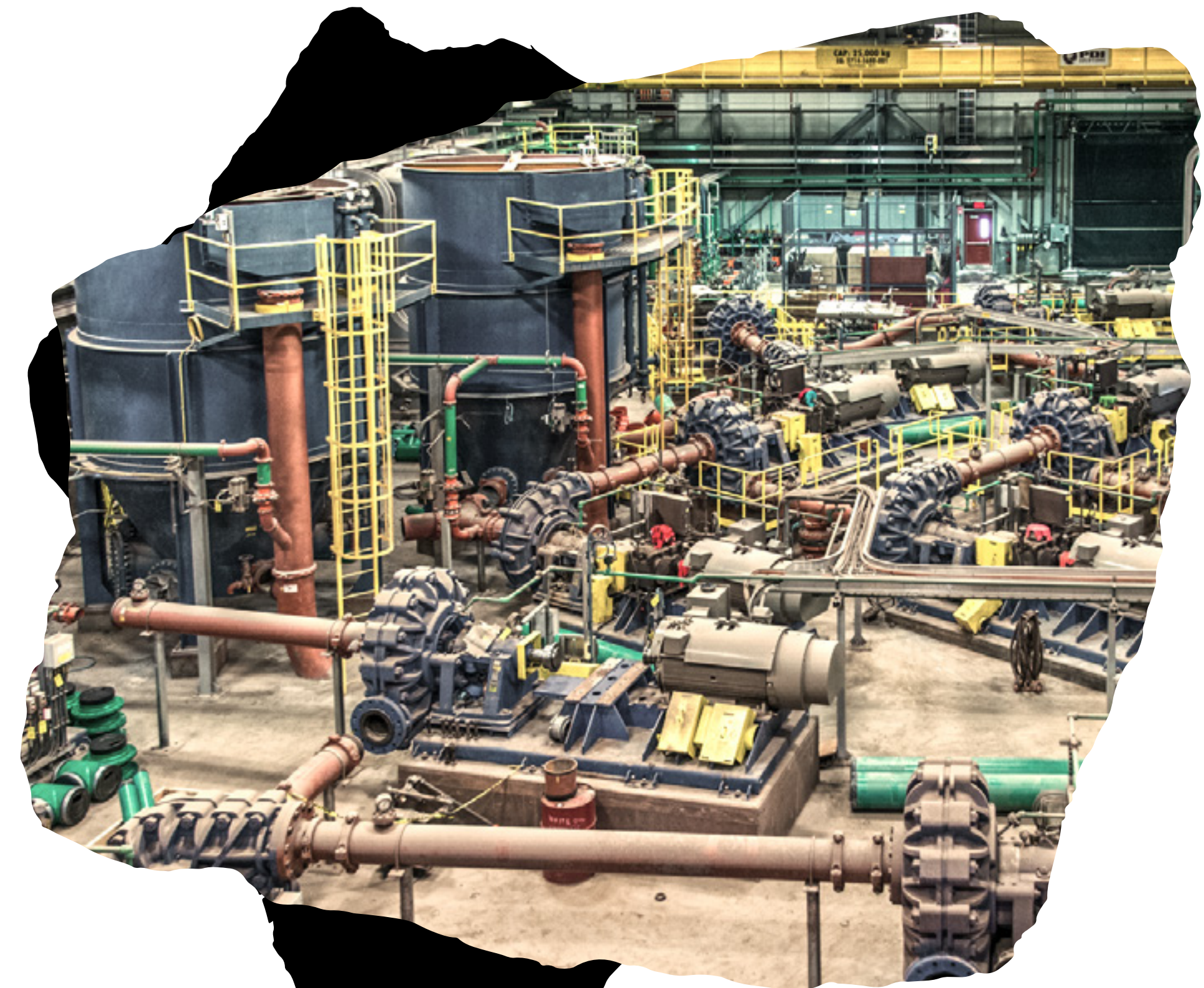
Booster station used to pump tailings
